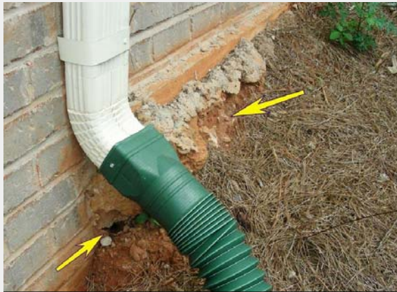
Erosion Under Foundation
