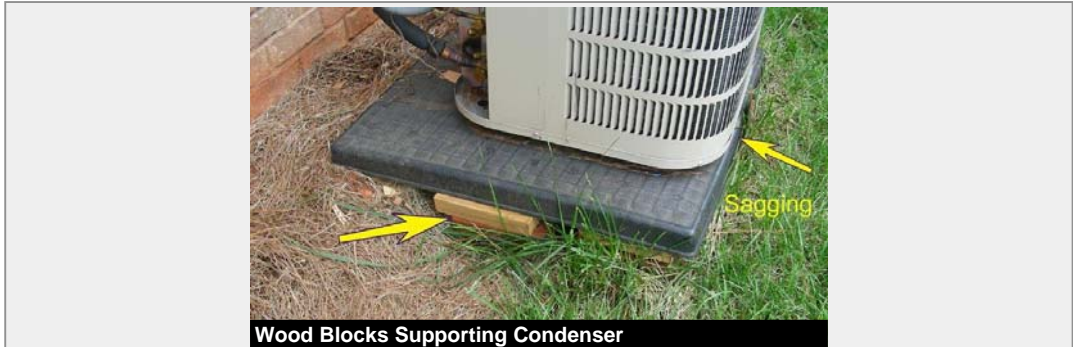
Wood Blocks Supporting Condenser
