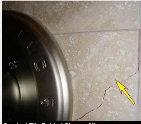
Cracked Tile Behind Shower Mixer
