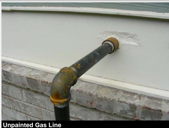
Unpainted Gas Line
