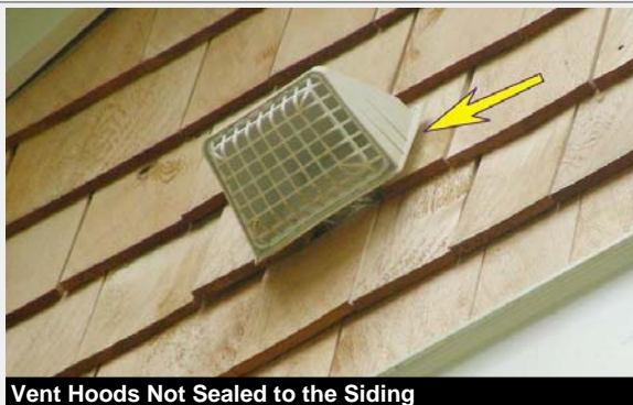
Vent Hoods Not Sealed to the Siding
