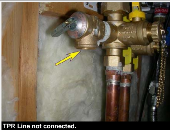
TPR Line not connected.
