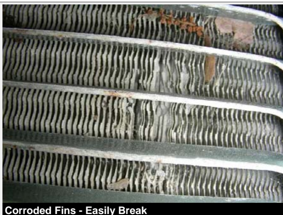
Corroded Fins - Easily Break
