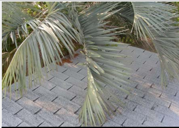
Trees Contacting Roof
