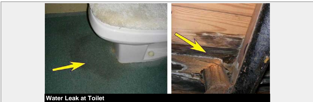
Water Leak at Toilet
