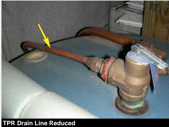
TPR Drain Line Reduced
