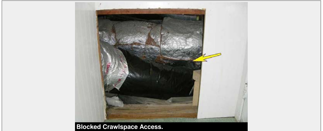
Blocked Crawlspace Access.
