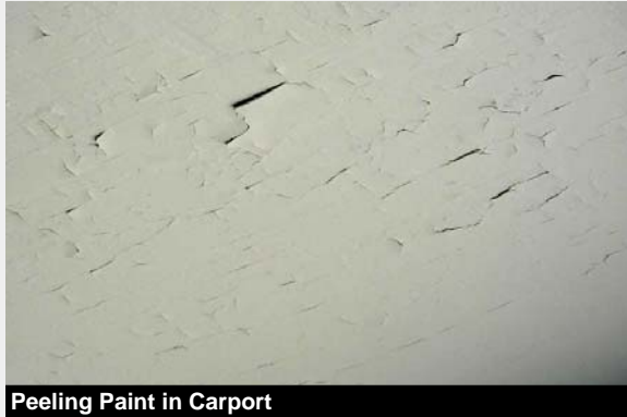
Peeling Paint in Carport
