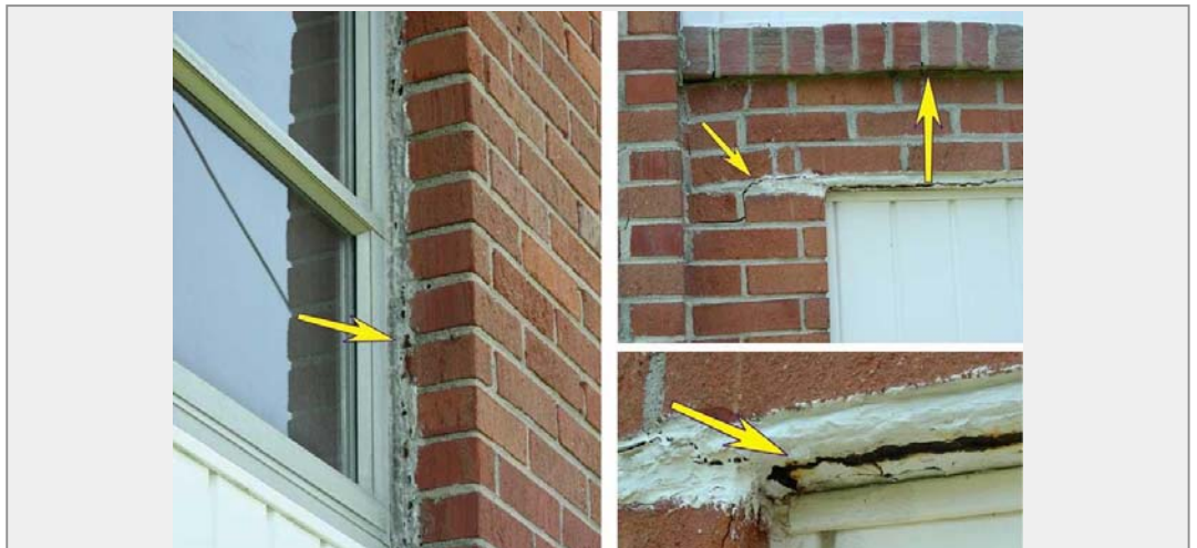
Bowed Brick / Rusted Lintel
