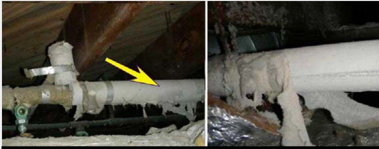
Possible Asbestos Insulation
