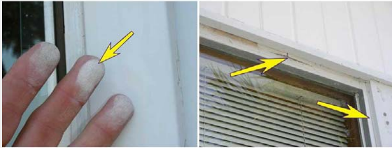
Worn Trim Paint / Sealing Needed at Joints
