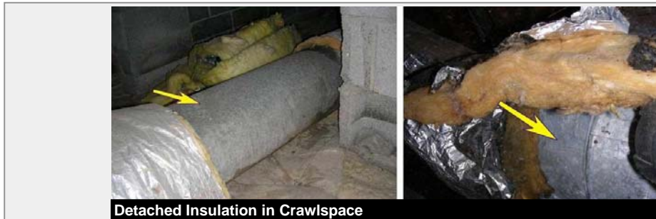
Detached Insulation in Crawlspace
